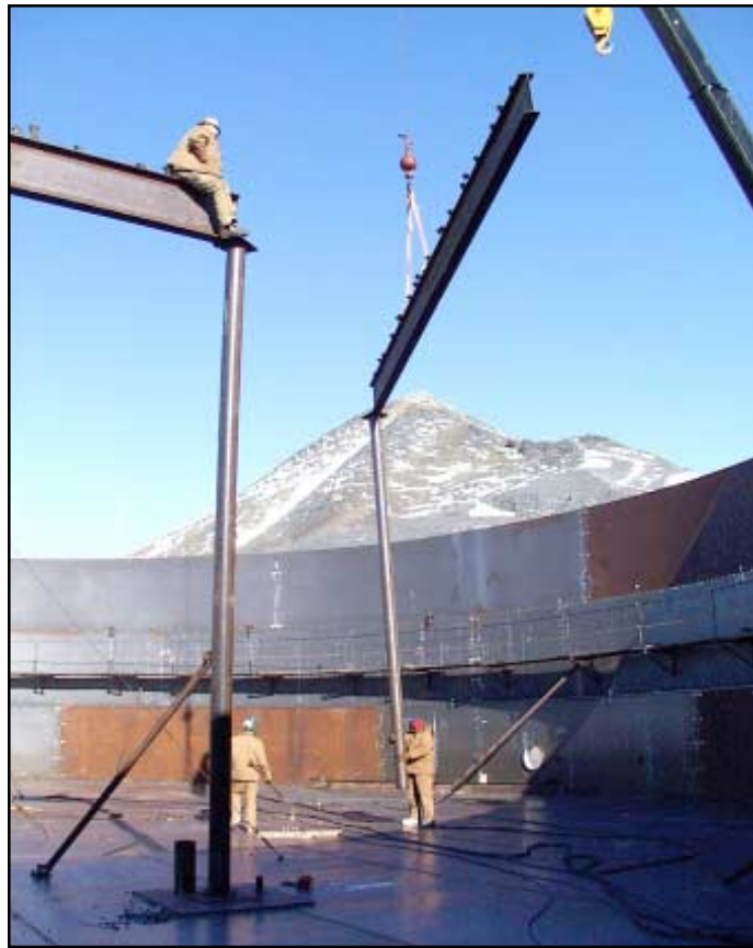
Rusty Baron guides a structural support into place for a new fuel tank as John Bray, Jr. and Tom Ehmstrom (seated above) get ready to fasten it in place. Photo by Josh Landis.
