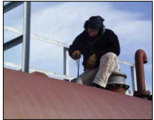
Brooke Grant checks the level of fuel in a tank as it refills. On an average flying day, the planes use about 50,000 gallons of fuel. Fuel is piped from the large tanks in McMurdo down to the ice runway to keep the planes supplied.
