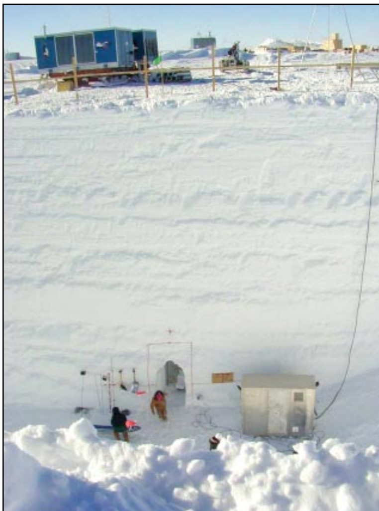
Ray Medina hauls a banana sled full of excavated ice out of a hand-dug pilot tunnel at the South Pole. The final corridor will be 2,000 feet long. Photo by Josh Landis.
