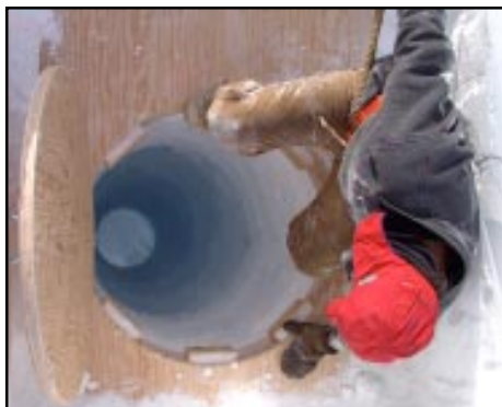
Mining foreman John Wright looks down an escape/service shaft for the new water and waste tunnel at the South Pole. Photo by Josh Landis.
