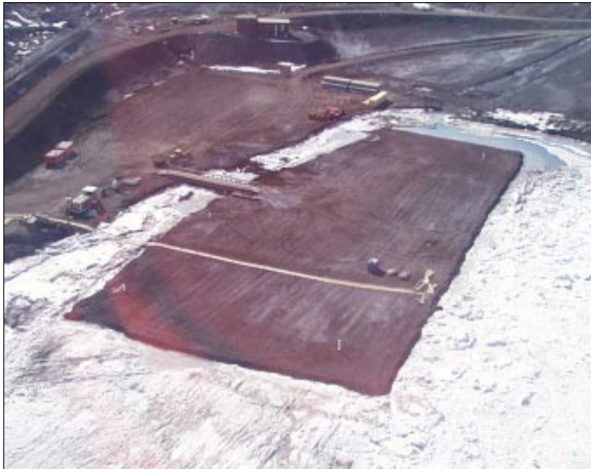
Construction on the ice pier began early in the winter season. Photo by Josh Landis.
