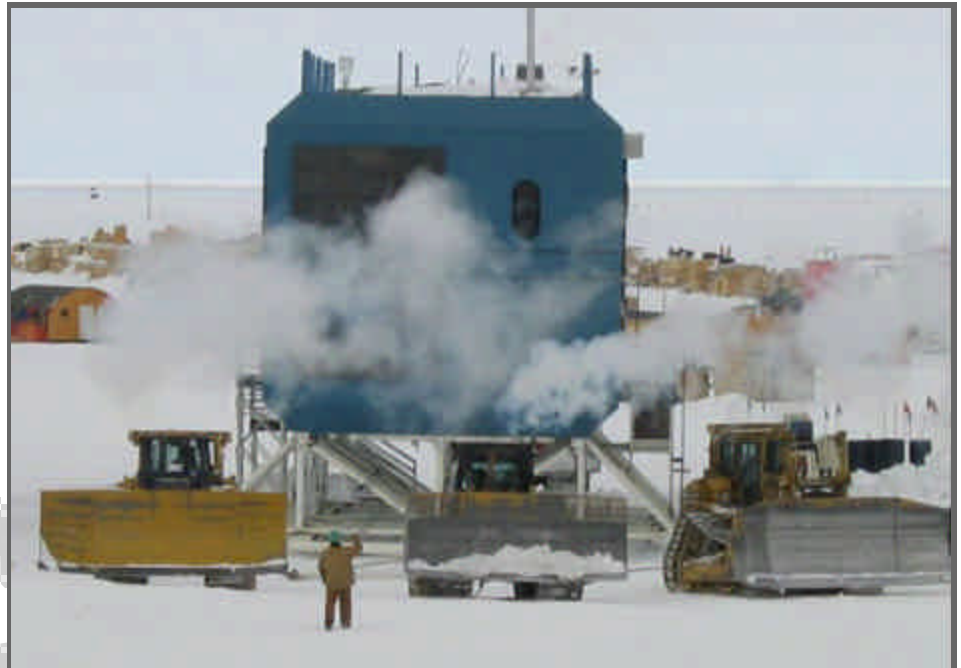
Photo by Mark Eisinger / Special to The Antarctic Sun Martin Lewis directs three bulldozers moving the El Dorm to a new location and a new purpose. The dorm will become laboratories for the IceCube science project.
