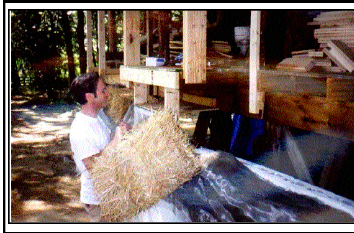
Greg Lehman sets a strawbale onto the foundation of his home in Goshen, Ind. He is building the house using environmentally-friendly methods and materials.
